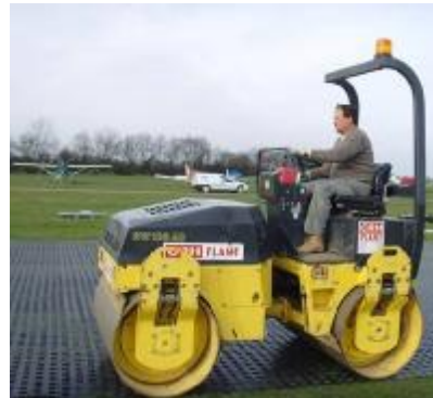
After about 3-4 rows are laid out, they should be rolled in leaving the last row unrolled.
